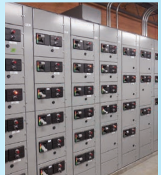
Honey Creek Feed Mill, PDC Electrical Contractors
