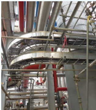
Badger State Ethanol Plant Expansion, PDC Electrical Contractors
