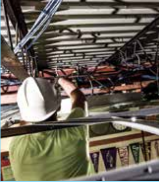
Delavan-Darien School District – Energy Efficient Lighting Upgrades / Faith Technologies, Inc.
