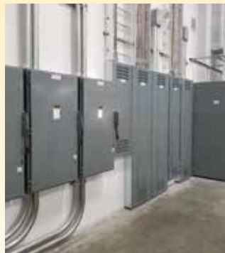
MGS Clean Room Steiner Electric, Inc.
