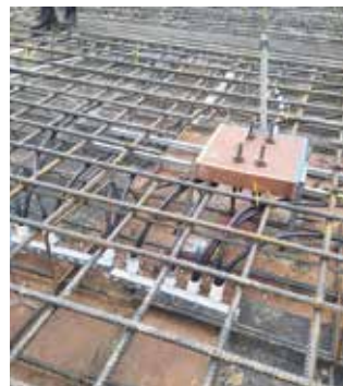
Exact Sciences Amenities Building North American Mechanical, Inc.
