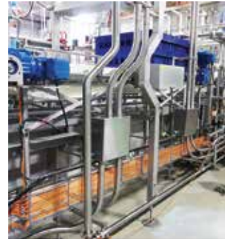
Klondike Cheese - Feta Cheese Line Expansion/Upgrade PDC Electrical
